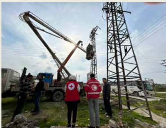
Working with the Syrian Arab Red Crescent, the International Committee of the Red Cross (ICRC) delivered a transformer to reinstate access to water for around 100,000 people. © ICRC
